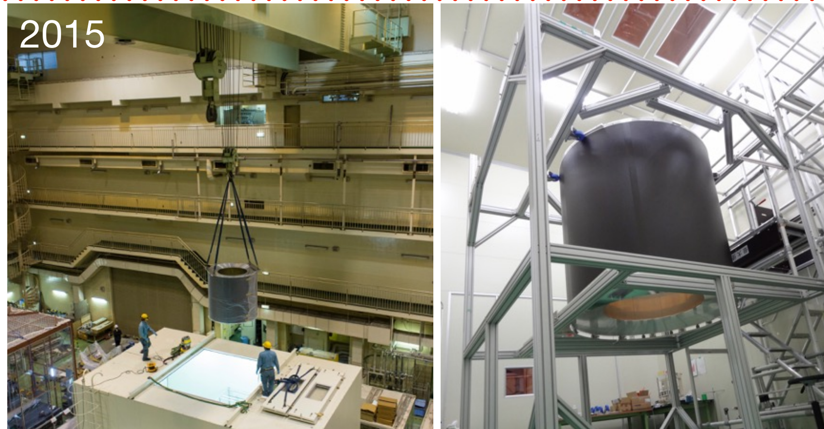
2015 Outer structure was transported to a KEK assembly hall, and set on a wire stringing cradle.
